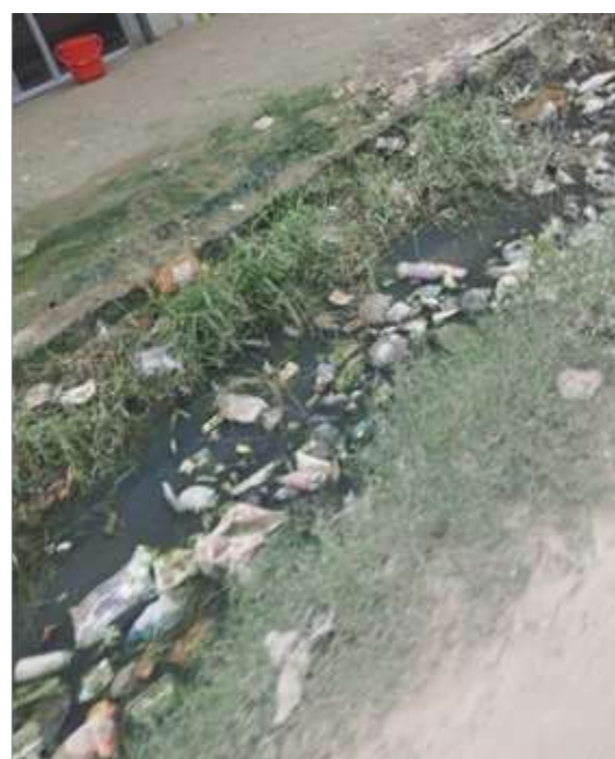
Recurrent blockage of secondary drains- Open drains carrying solid waste
