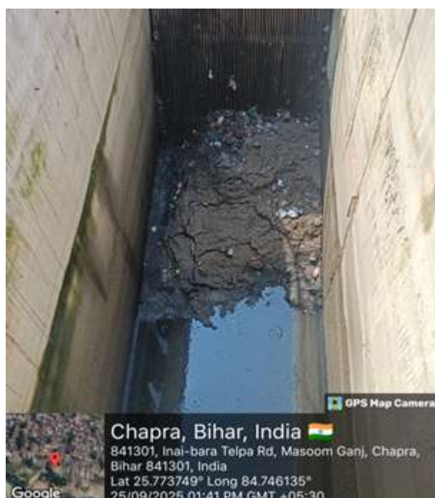
High siltation- leading to infrastructure failure
