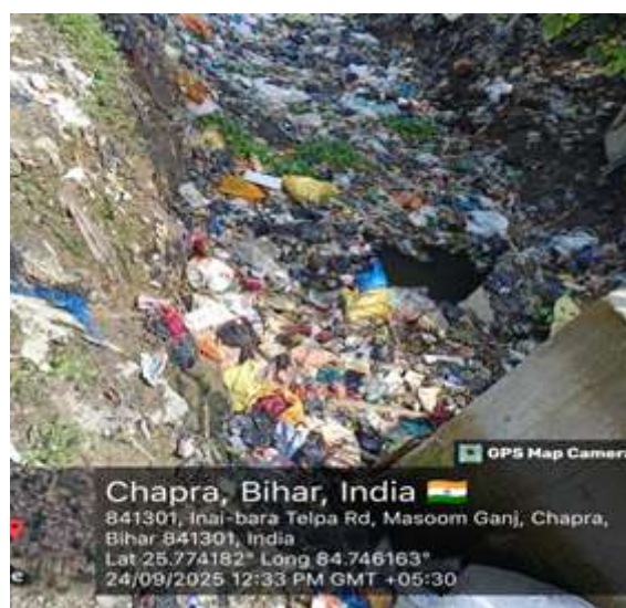
Solid waste accumulated at outfall points towards river
